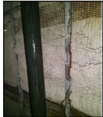
Example of condensation on the cold-water riser.
